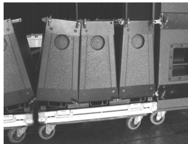
(vi) All dV-DOSC attached at front, in blocks of 3 at the rear (except for dV-DOSC #1 to #2)
